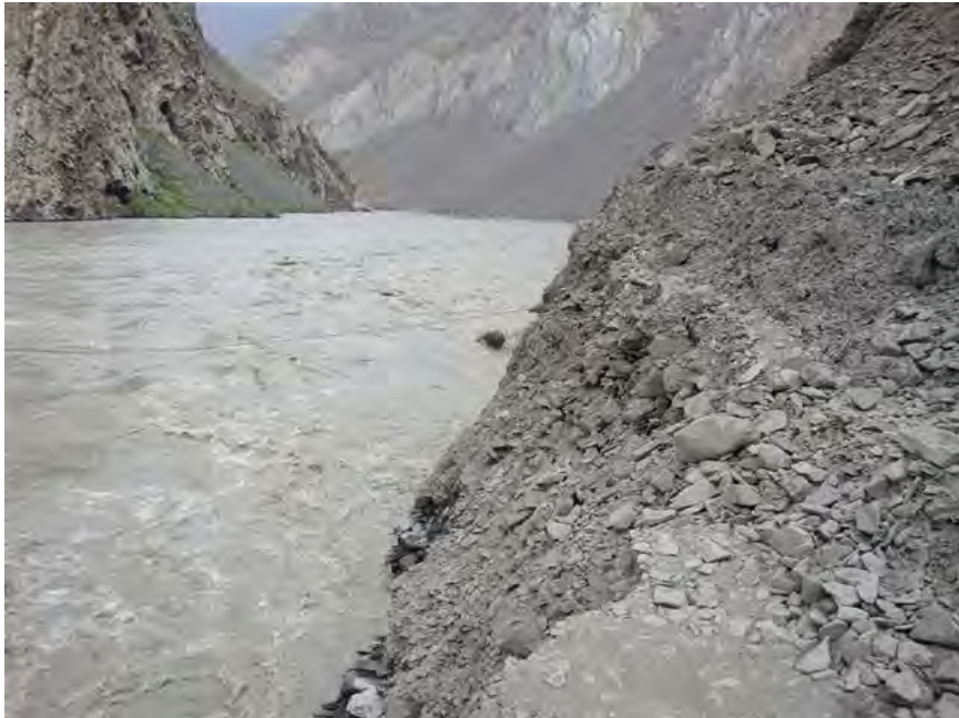
Collapsed cliffside road near Roshorv in the Bartang valley, August 2010 (Stéphane Henriod)
