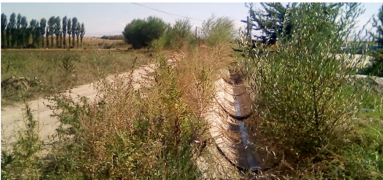
Figure 4. View of the rehabilitated part of the 1-2 Maya canal by reinforced concrete trays
